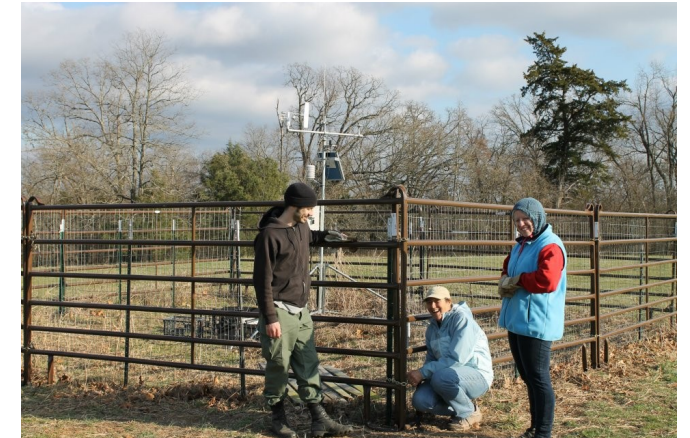
Andre Bresson, Celeste Prussia, Tara Elmore, and Janice Greene (behind the camera) repair the fence around the weather station damaged by the elk herd in Drury Conservation Area
